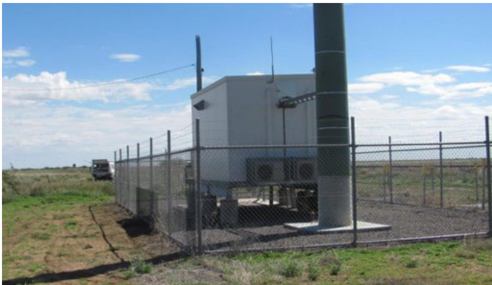
Plate 18-3 Typical CEV hut
