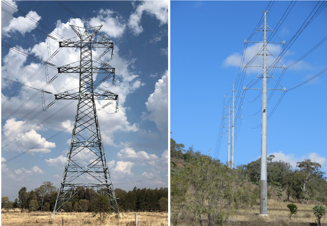
Plate 18-1 Typical 330 kV double circuit steel lattice transmission tower (left) and 330 kV double circuit monopole (right)
