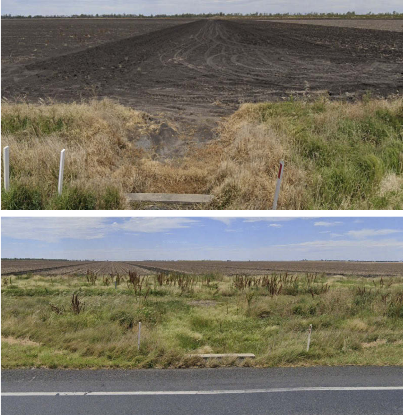
Figure 3.10 Culvert on the Gore Highway at approximate chainage 145 km. Upper image is looking upstream, silt from bare cropland upstream has been deposited near the inlet, the grass buffer is less than 10m at the time of the photo. Lower image is looking downstream, wide grass buffer between culvert outlet and crop, approximately 40m. The small bare patch roughly halfway between the culvert and crops is a farm track.
