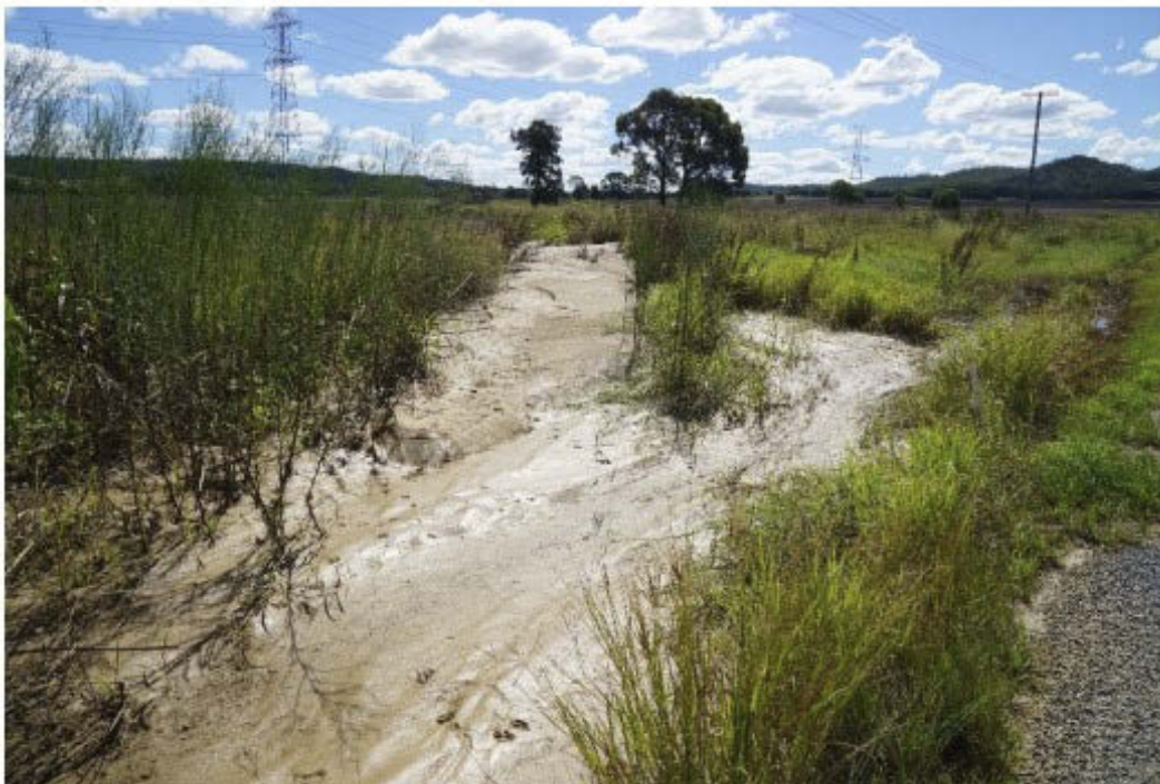
Figure 3.25 Site 7a – SC 6, deposition has blocked culvert and caused deposition and ponding, indicates erosion occurring upstream of site
