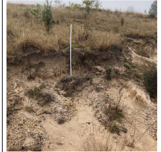
P8 – bank erosion on true left, downstream of culvert, white staff for scale 1.0 m (site E12)
