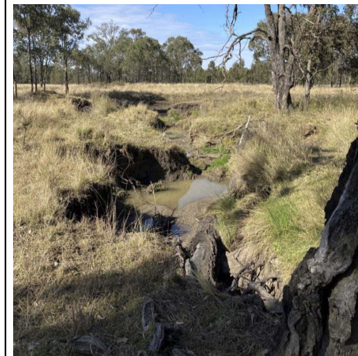
P16 – bank erosion downstream of road culvert (site E4)
