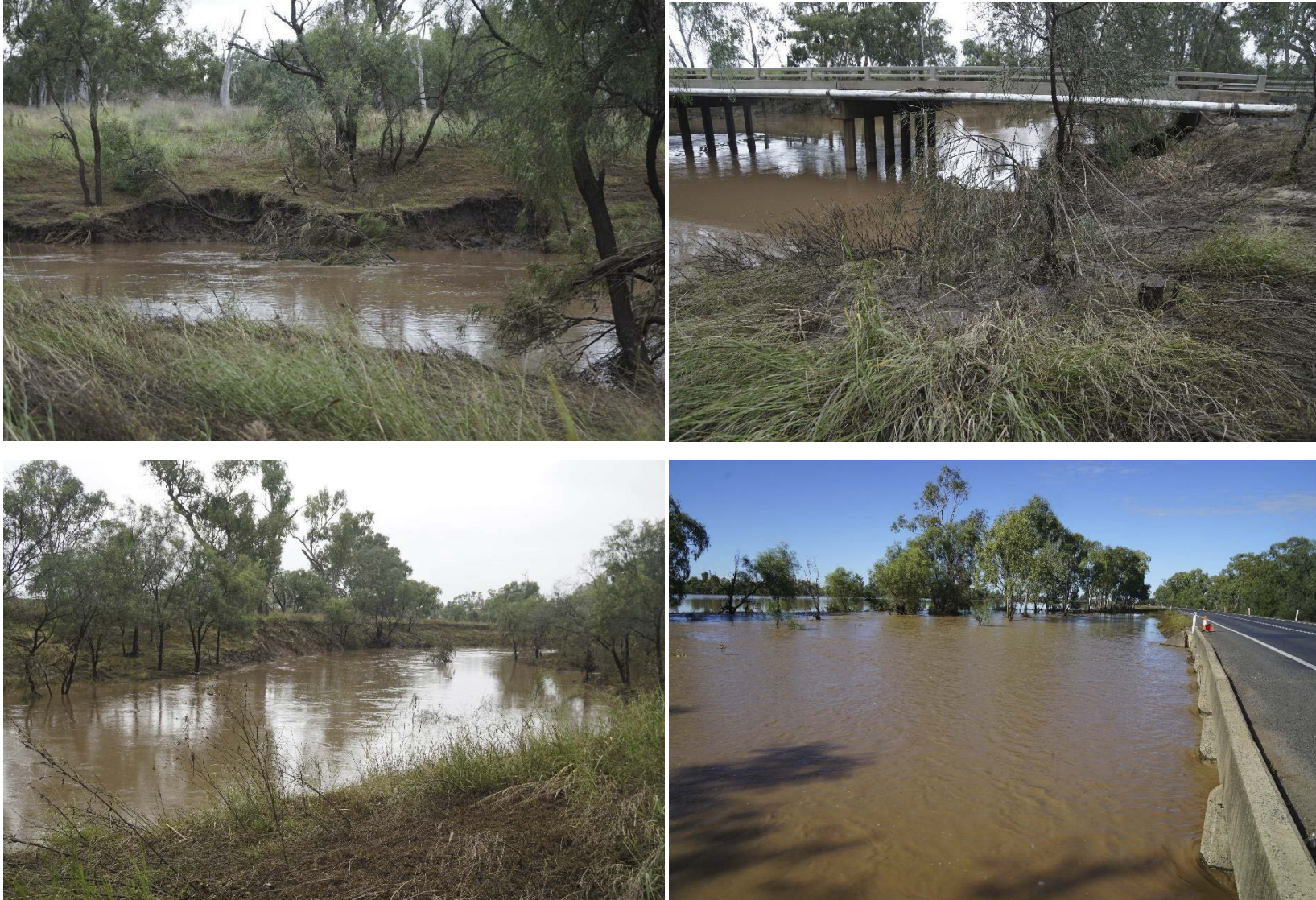
F. 3 Site 1d/EP16 photographs. Downstream failures (top left), bridge from downstream side (top right), from upstream left bank (bottom left), true left upstream (culverts underwater) (bottom right)
