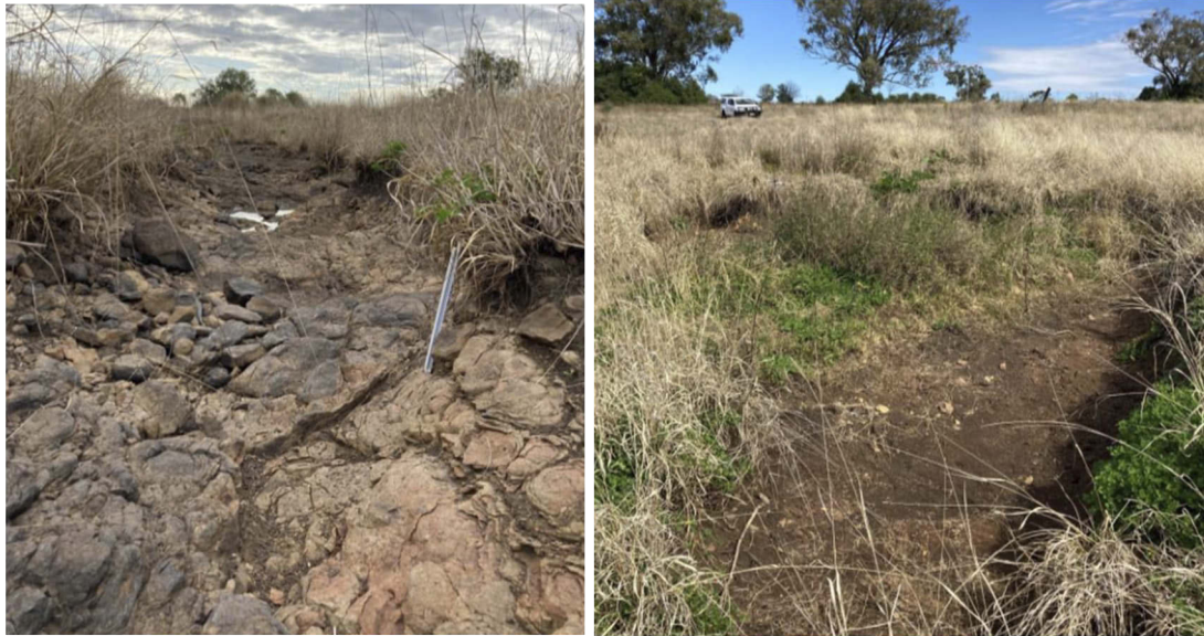
Figure 1 NC 11 site photos. Left, Photos P9 – rock channel near design culvert. Right, Photo P10 – minor erosion (erosion site E2) in the silty clay channel bed, 1 m drop in bed level directly upstream of this erosion. See Appendix A drawing E3 for photos locations and descriptions.
