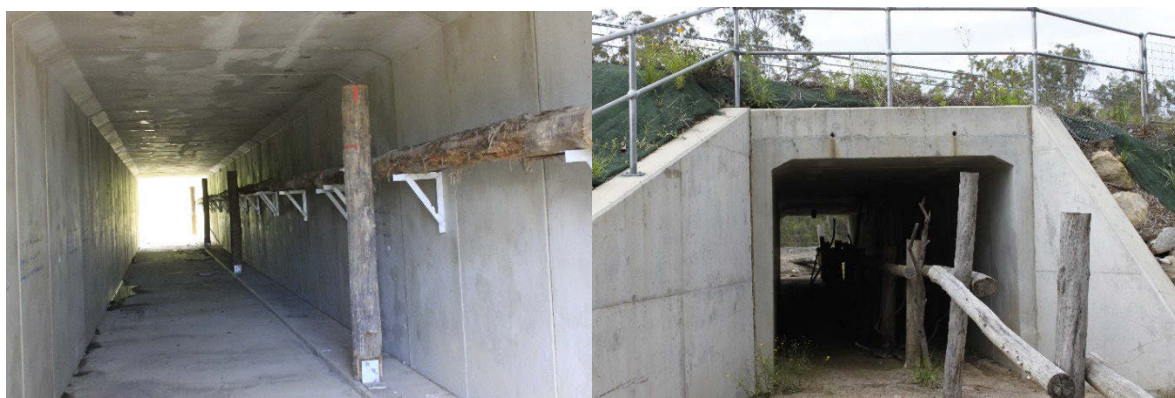
Figure 5.14 Koala rails in culverts under the Pacific Highway, Woolgoolga to Ballina. The installation on the left has a concrete floor, and the rail is attached to the wall with brackets and climbable posts secured to the floor and the rail. In contrast, the installation on the right has an earthen floor and the rail is stand-alone. In both cases, the post does not interrupt movement along the rail. Photos: Rodney van der Ree.
