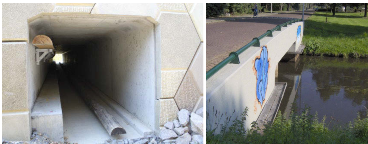
Figure 5.7 Example of strategies that provide dry passage if the culvert contains standing or flowing water. Note that the concrete ledge and timber shelf in the left photo are still to be connected back to the adjacent habitat. Photos by Rodney van der Ree WSP.
