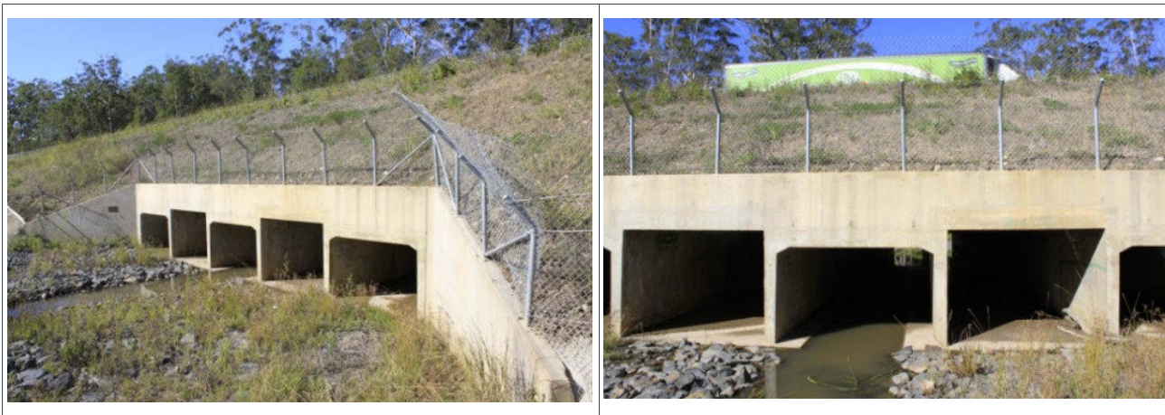
Figure 5.6 Example of multi-cell culverts on the Pacific Highway NSW where the middle cell is designed to take water flow year-round, with the outer cells remaining dry except during flood events. Photos Rodney van der Ree WSP.
