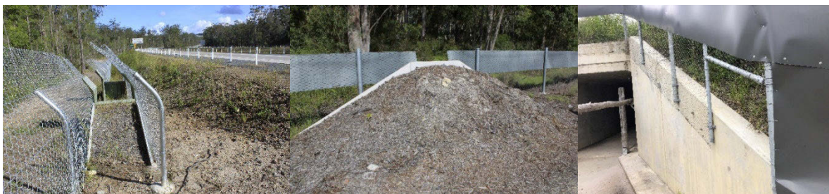
Figure 5.17 Jump-outs for Koalas on the Pacific Highway, including two options for a ramp on the road-side of the fence (left and middle) and integrating the jump-out with the wing-wall of a wildlife culvert (right). Photos Rodney van der Ree (left and middle) and TfNSW (Right).
