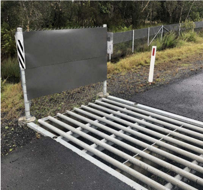
Figure 5.16 Koala grid at Evans Head, New South Wales (Source: TfNSW).
