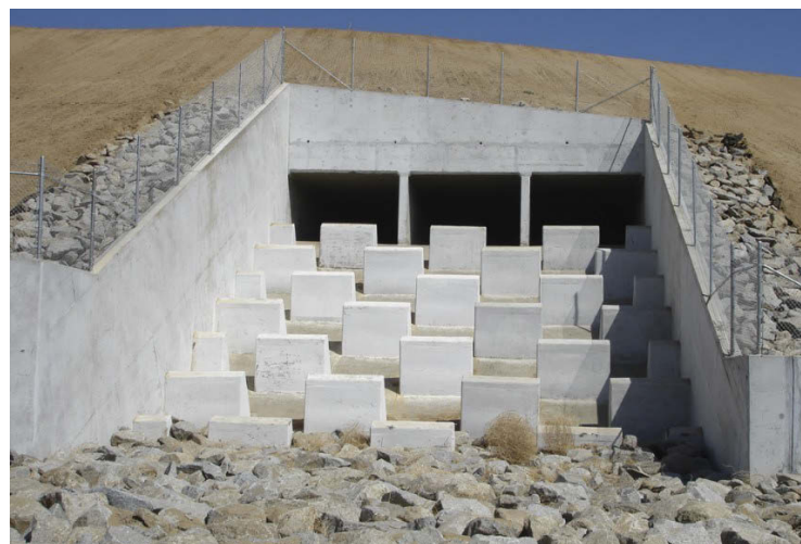
Energy dissipater to reduce velocities (PACE Advanced Water Engineering)
