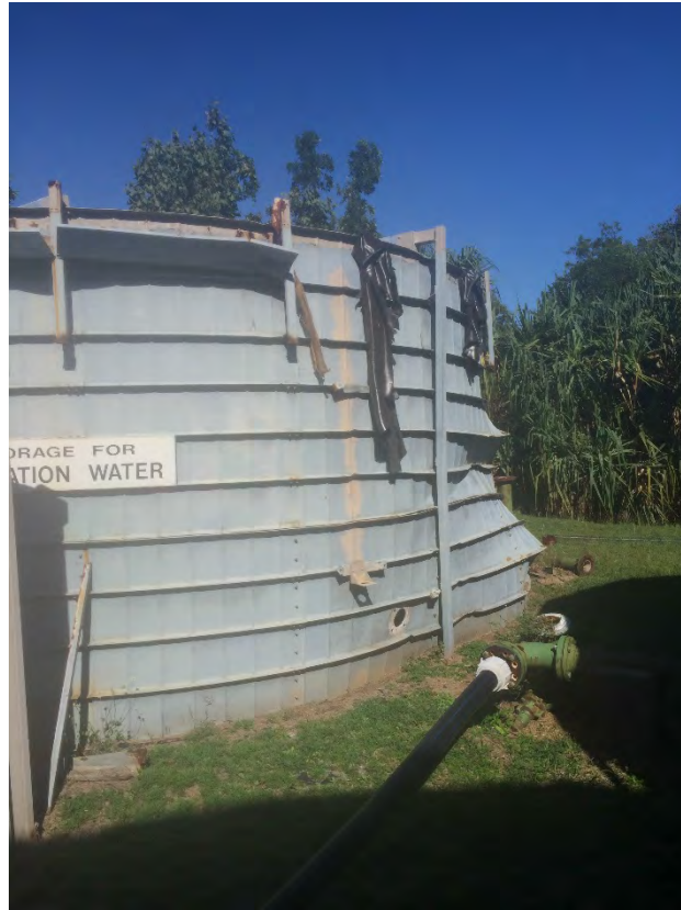
Photo 5: Burst water storage tank
