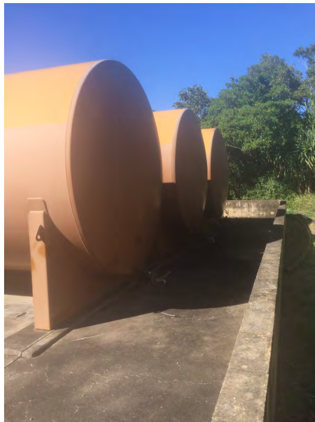
Photo 6: Fuel tanks in bunded area
