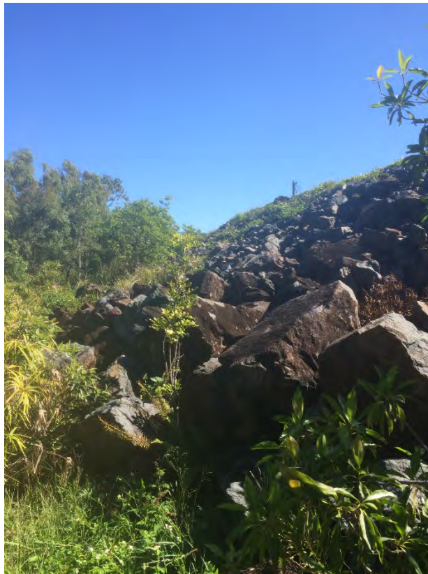
Photo 12: Downstream dam wall with tree growing
