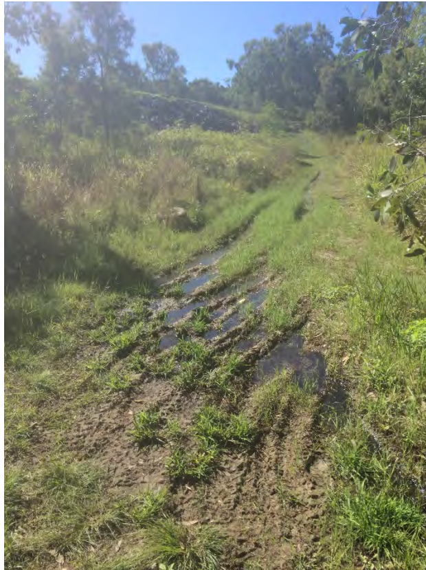
Photo 11: Dam downstream wall with seepage area
