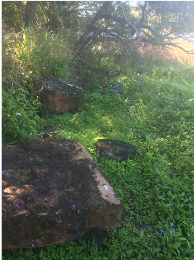
Photo 7: Boulder and vegetation in dam spill way
