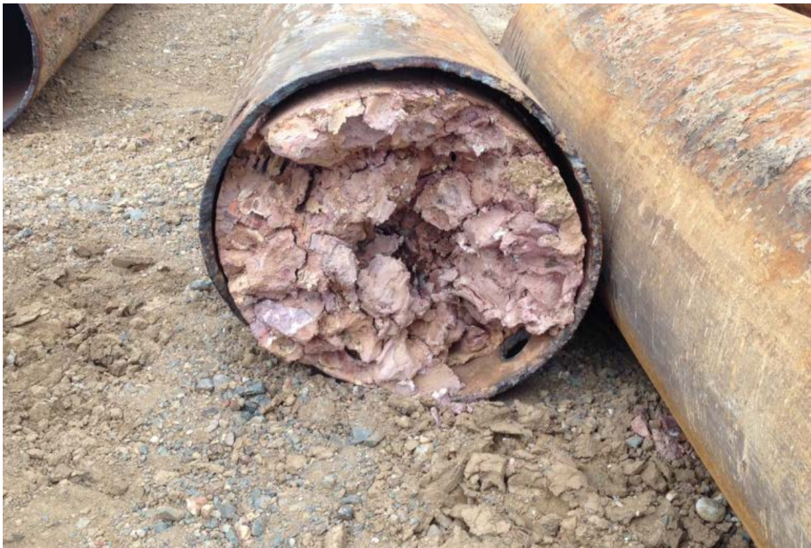
Figure 5.4 Sinker pipeline blockage during the Western Basin Project dredging (pipe diameter shown is 900 mm)
