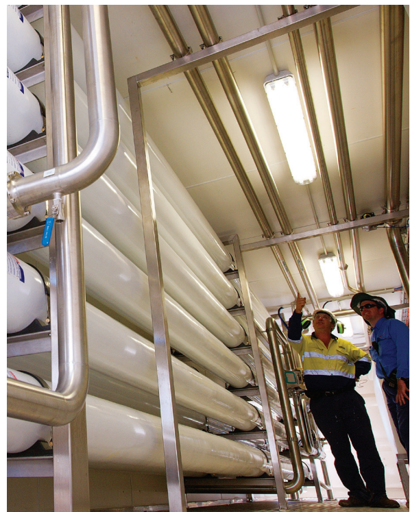
Reverse osmosis facility.
