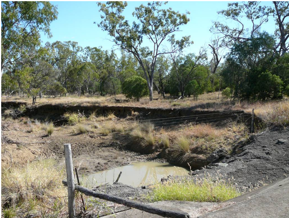
Plate Pipeline 63. Roche Creek in Segment 21 west of box culvert on northern channel showing scouring and bank erosion (55J 798390E 7119980N)
