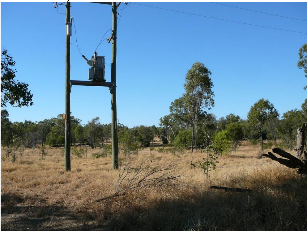
Plate Pipeline 34. Pole-mounted power transformer in wide road reserve in Segment 15 (56J 311030E 7149260N)
